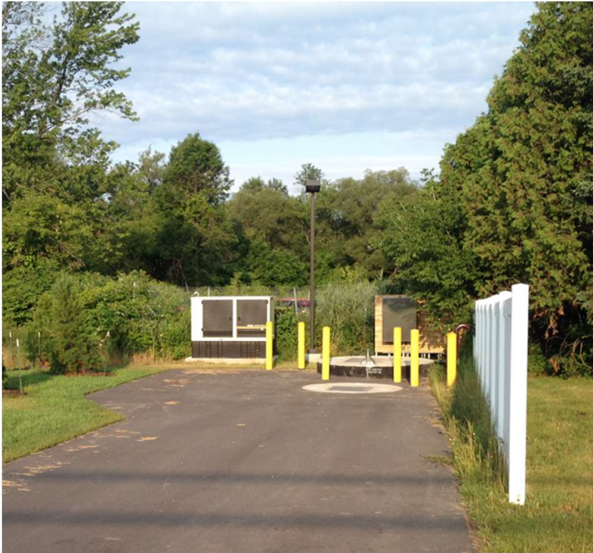
Pump Station – below grade with emergency generator and control panel
